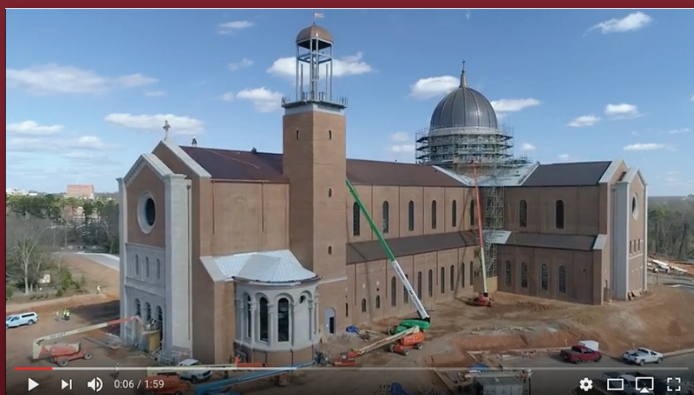
■ Cathedral tour – See the detail – from columns to the glowing copper roof. Flyboy Photo and Media in Raleigh delivers a tour of the Holy Name of Jesus Cathedral construction site.
